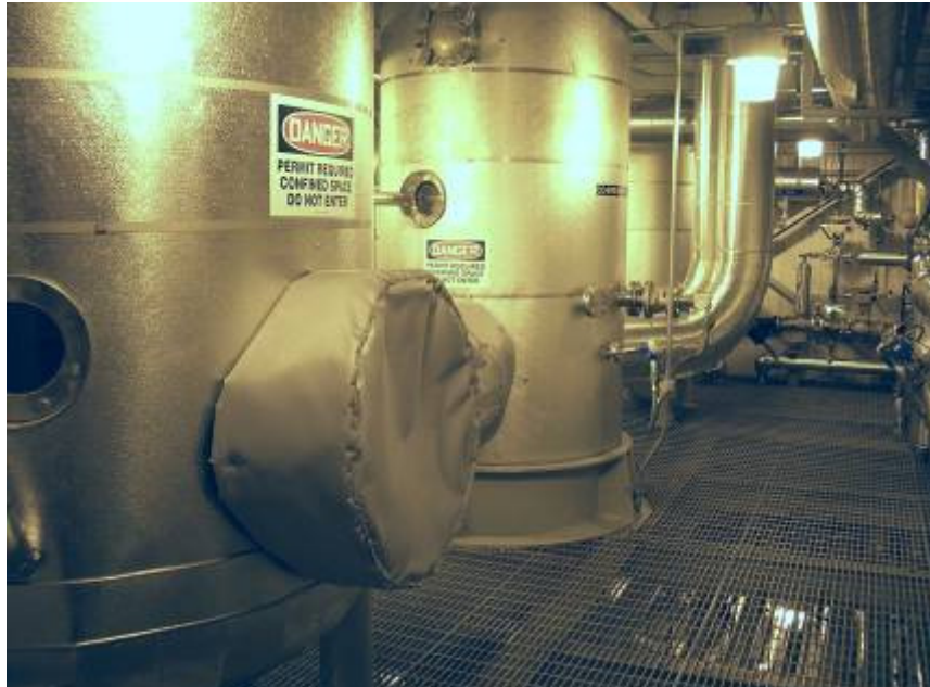
Cyclodextrin production at Eddyville (USA)
