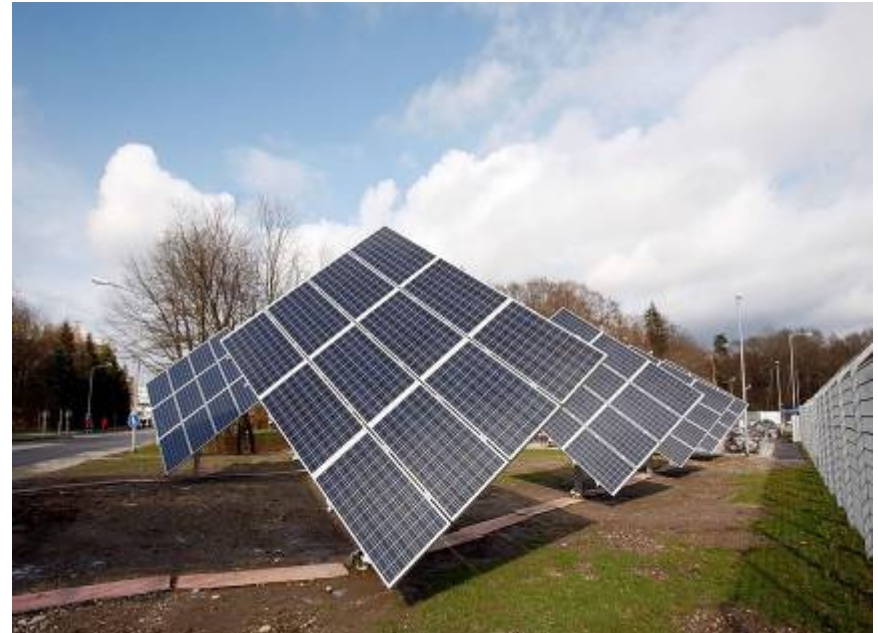
Solar installation at the Burghausen site
