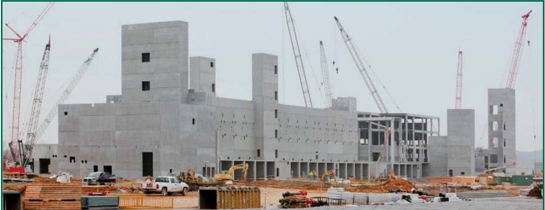
Deposition reactor hall for polysilicon production
