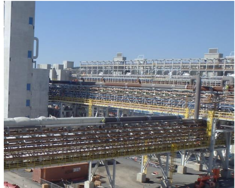
Hydrogen Recovery Unit
