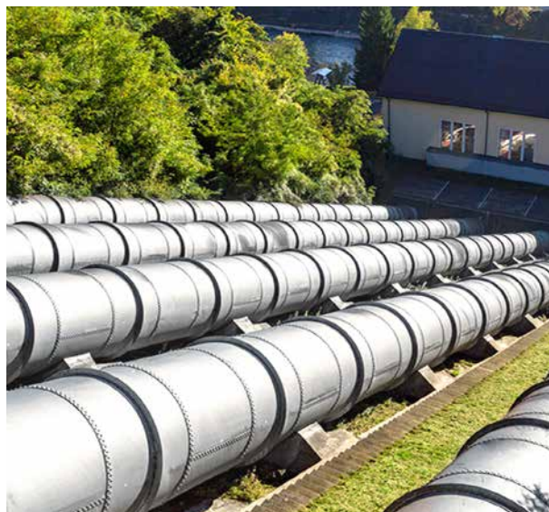
B I The Alzwerke power station has been supplying WACKER’s Burghausen plant with hydroelectricity for more than 100 years.
