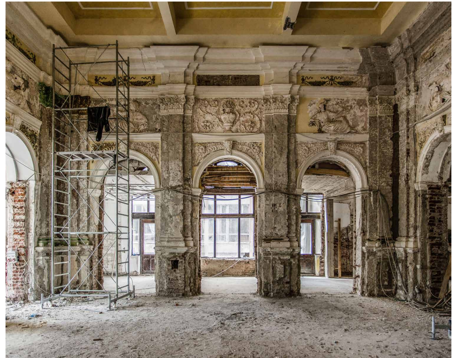
Past splendor: view of the interior of the casino, which was built in 1872.
