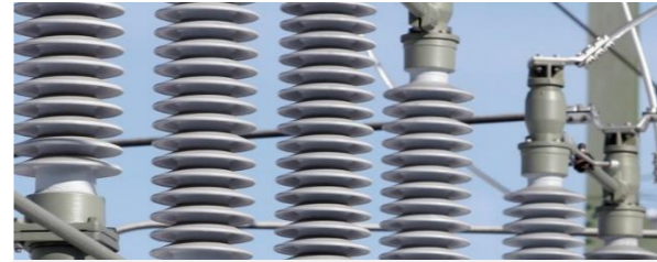
Insulators and cables
