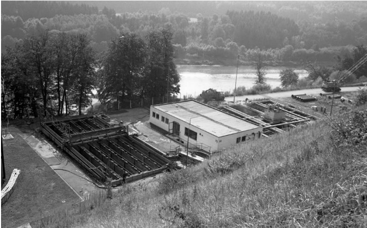
Caption: Milestone in the history of WACKER's industrial wastewater treatment: construction of the biological wastewater treatment plant (BARA) in 1974.
