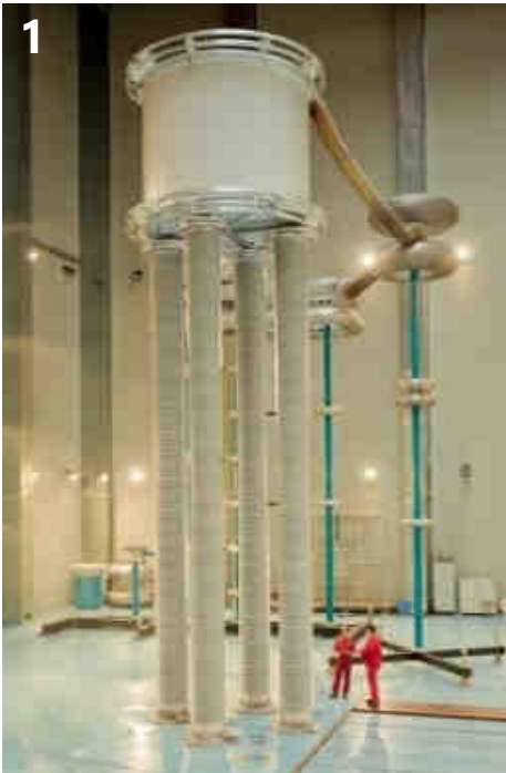
1 | CHSP (gas-filled) – coil support insulators
