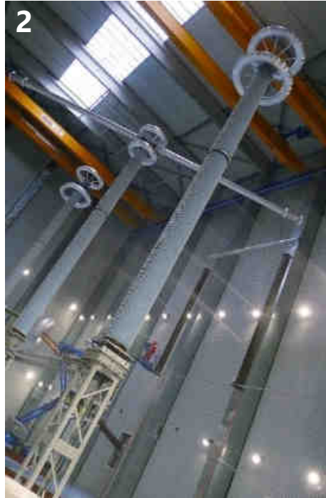
2 | 1.100 kV UHV disconnector
